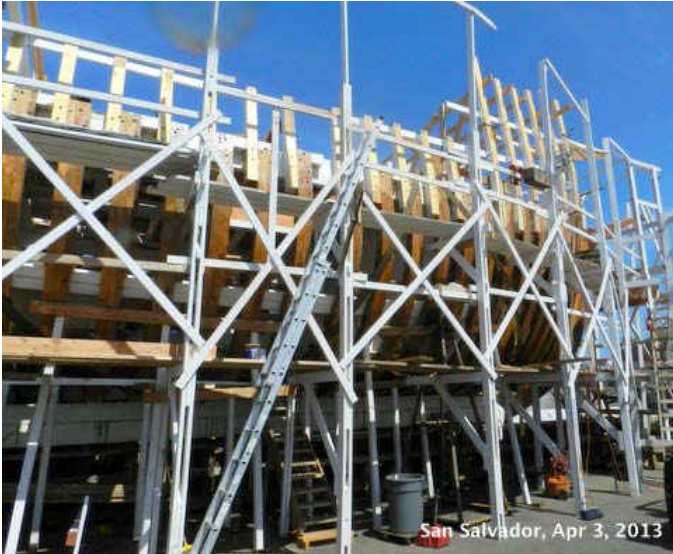
Looking toward the bow, stanchions for deck railing and forcible are in place.
